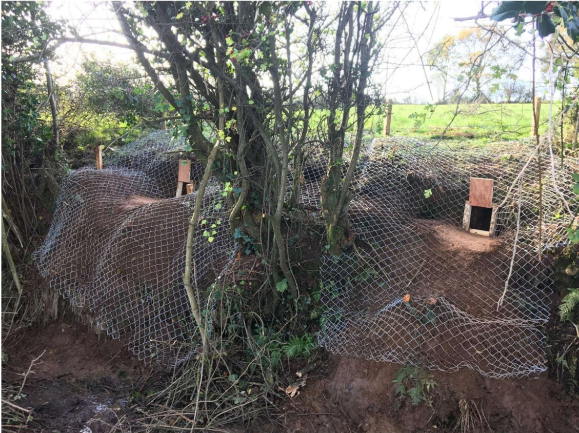
Plate 6-23: Example of One-way Badger Gates With Chain Link Fencing to Prevent Badgers From Digging Around Closed Entrances
